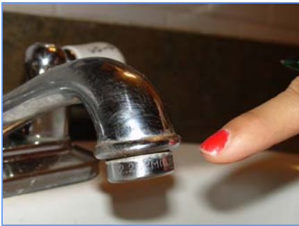
A Rahway High School Student notices that one of the school's faucets uses 2.22 gallons of water per minute.
